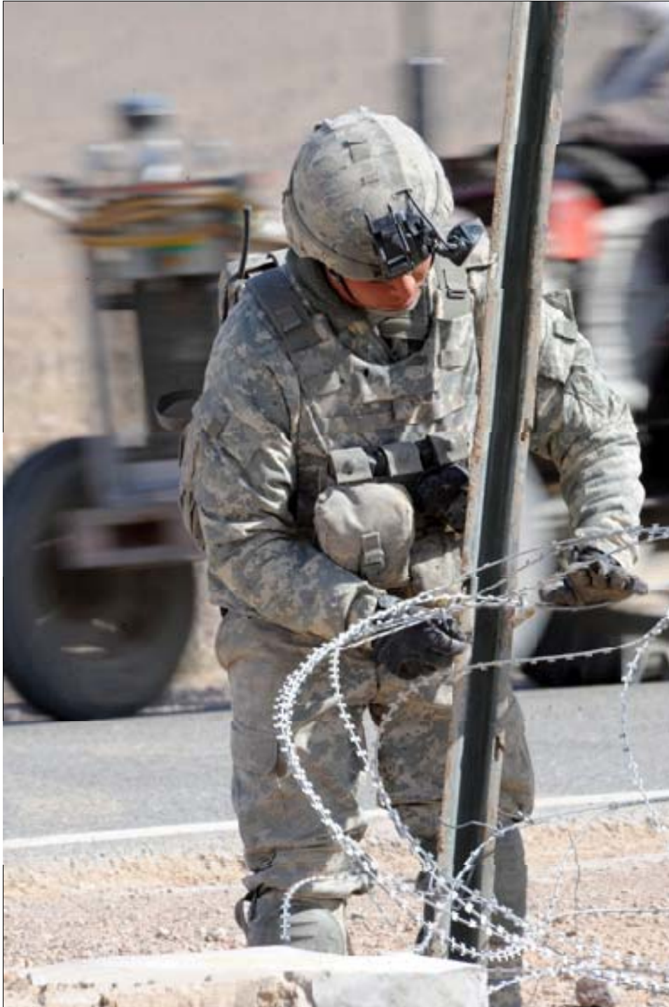
U.S. Army Staff Sgt. David C. Beyl with 8th Squadron, 1st Cavalry Regiment secures razor to a picket during a culvert denial operation along Highway 4, Spin Boldak, Afghanistan, Feb. 17, 2010. (U.S. Air Force photo by Tech. Sgt. Francisco V. Govea II/Released) (100217-F-9891G-108)
