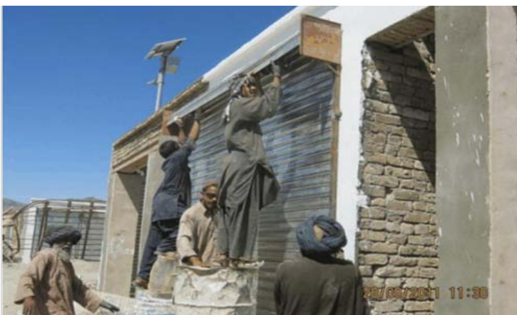
CDP laborers install roller doors that just arrived on US Marine convoy on shop front in Naw Zad bazaar.
